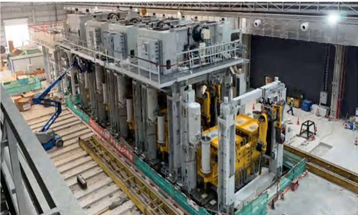
GIGAFACTORY SHANGHAI - MODEL Y FACTORY INTERIOR
